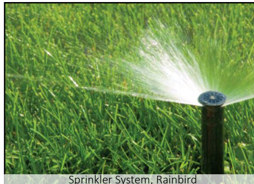
Sprinkler System, Rainbird
